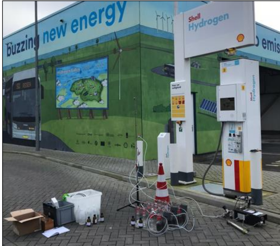
Commissioning H2 fuelling station
